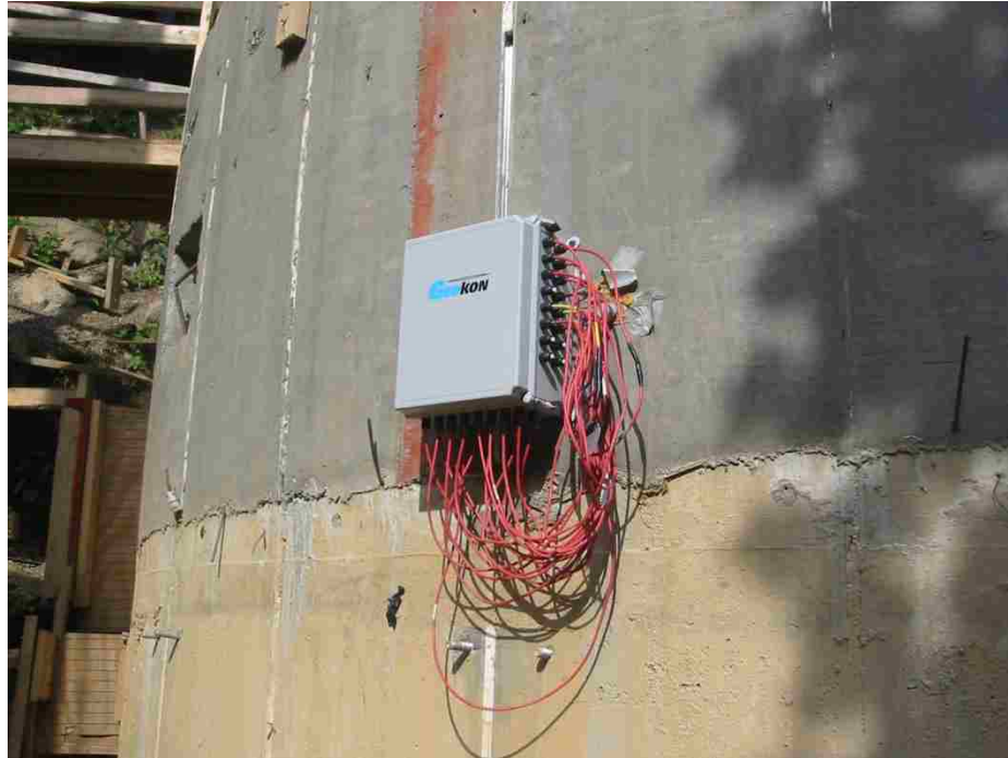
Figure 6.11. Photograph of Installed Terminal Box (Step 7)
