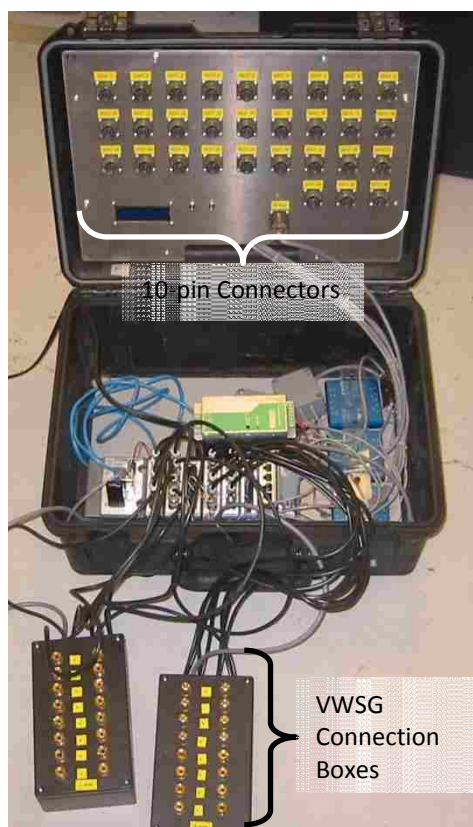
Figure 3.17. Photograph of Data Acquisition Box
